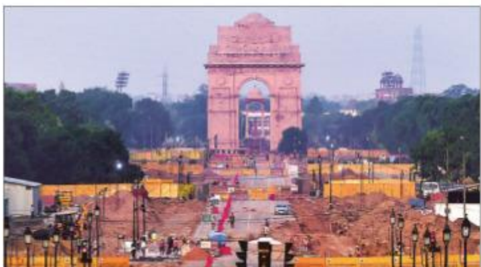
Construction work underway as part of the Central Vista project at Rajpath in New Delhi on Friday
